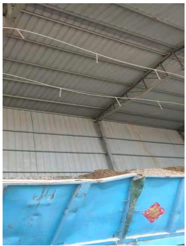
搅拌车间水喷淋
